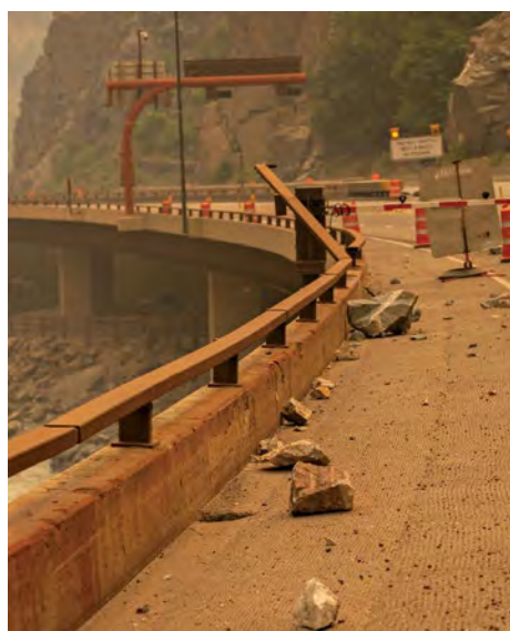
Falling rocks damage Interstate 70 during the 2020 Grizzly Creek Fire. Photo: Tom Story/USDA Forest Service Rocky Mountains
