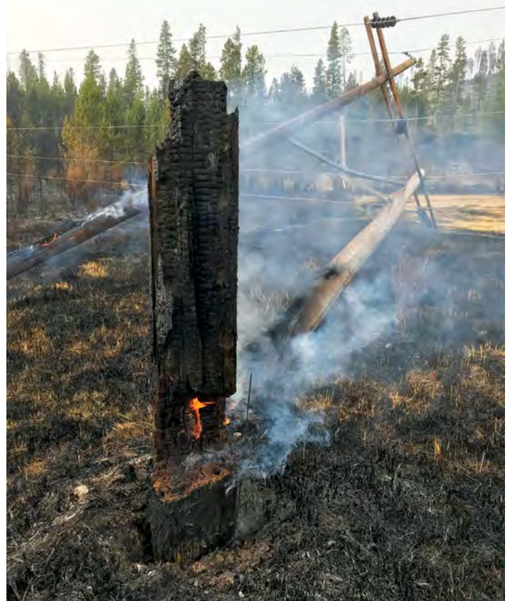
Several electric transmission line were damaged or destroyed by the East Troublesome wildfire. Photo: Ron Burbridge/Western Area Power Administration, ©CC2.0
